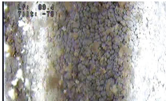
Deposit inside casing
